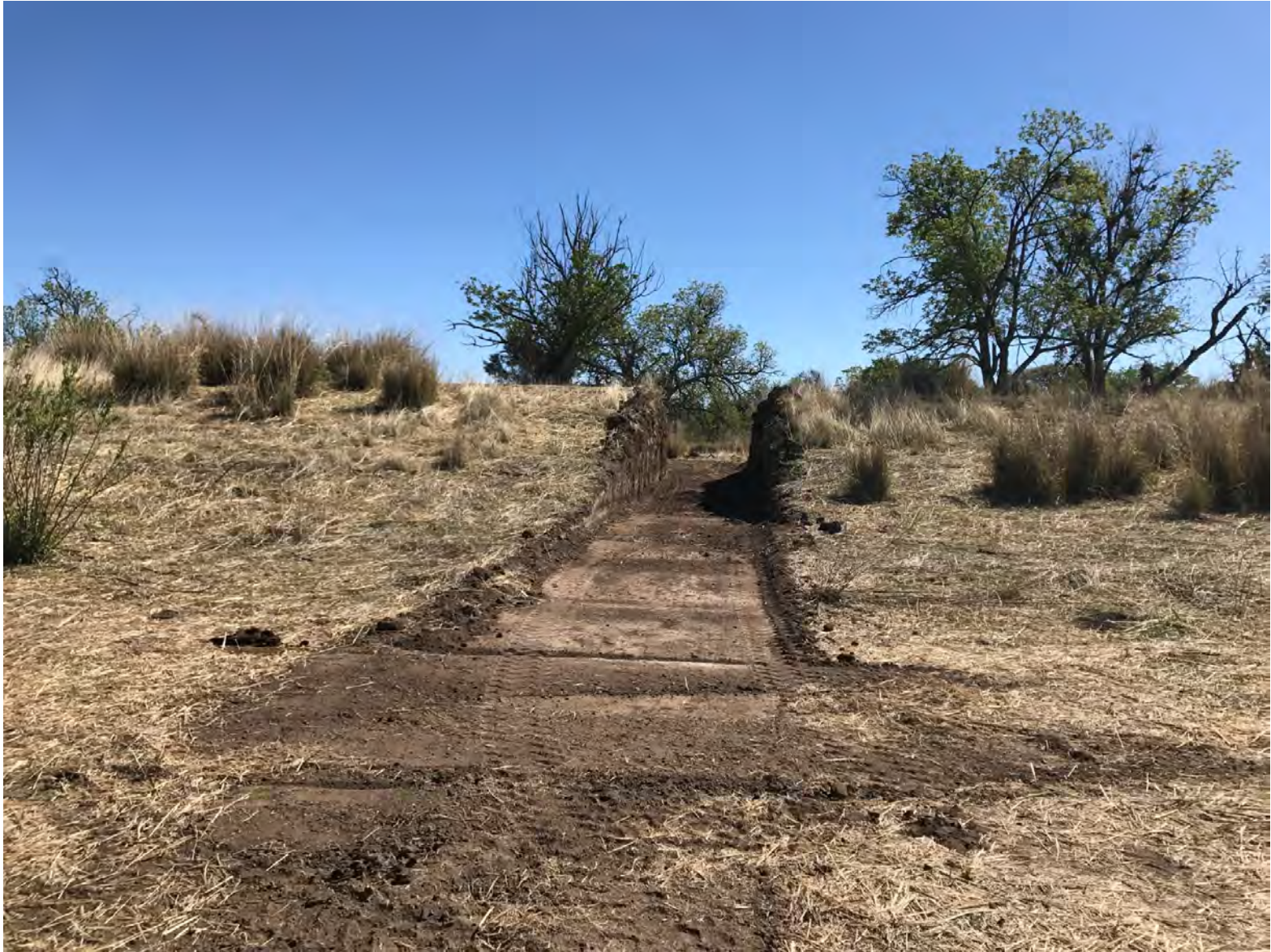
Levee cut on Diamond C Ranch-O'Donnell Canyon Ciénega
