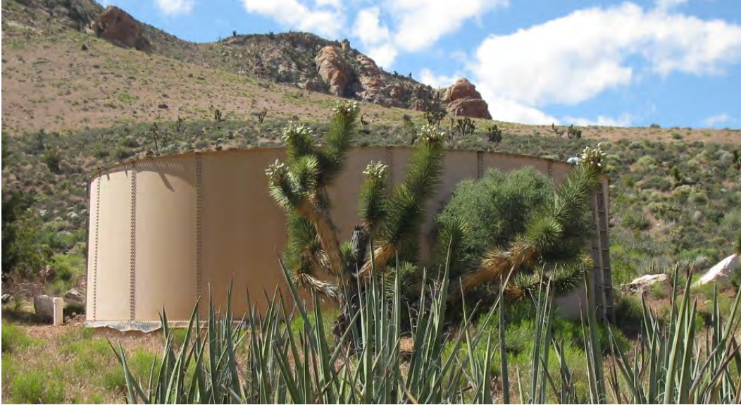
Figure B.3. Metal Storage Tank.
