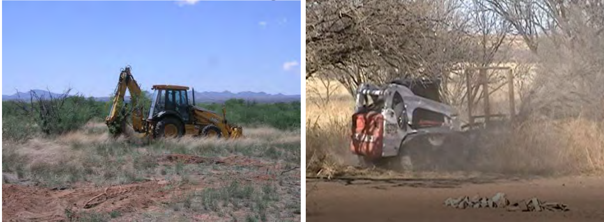
Figure C-1. Left: Mechanical Grubber (Tiller et al. 2012), Right: Masticator at work in the Airstrip (2017)
