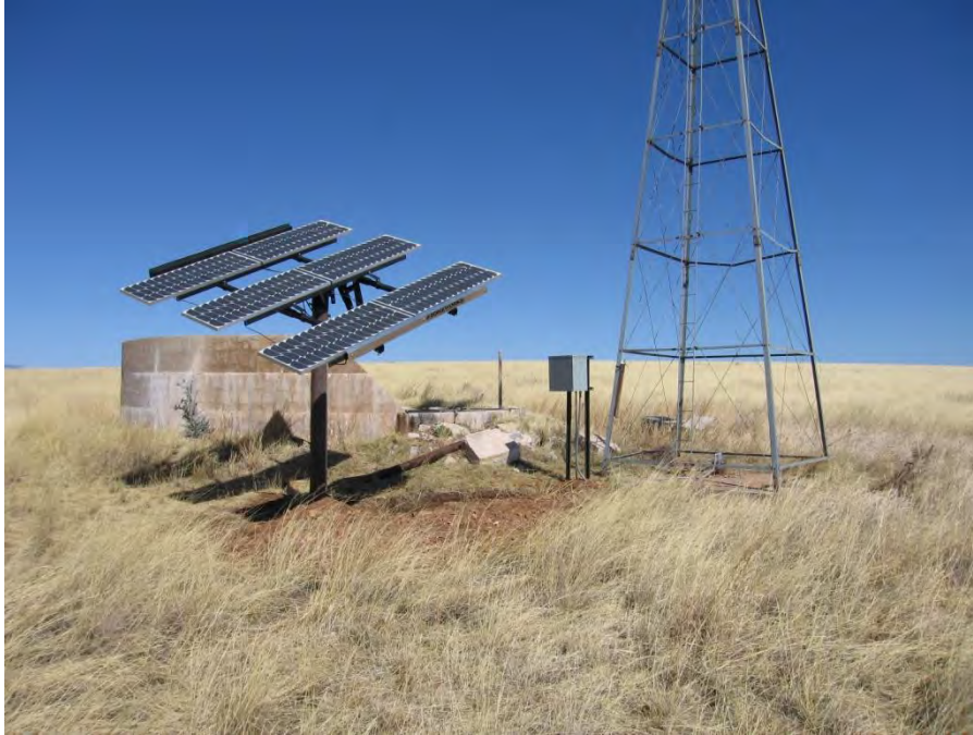
Figure 5. Example of solar system used to power well pump at Bald Hill Tank.
