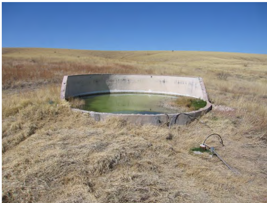
Figure 4. Photo of storage tank modified for wildlife water and aquatic habitat suitable for native fish and frog conservation at Antelope Tank. Note well in the foreground.
