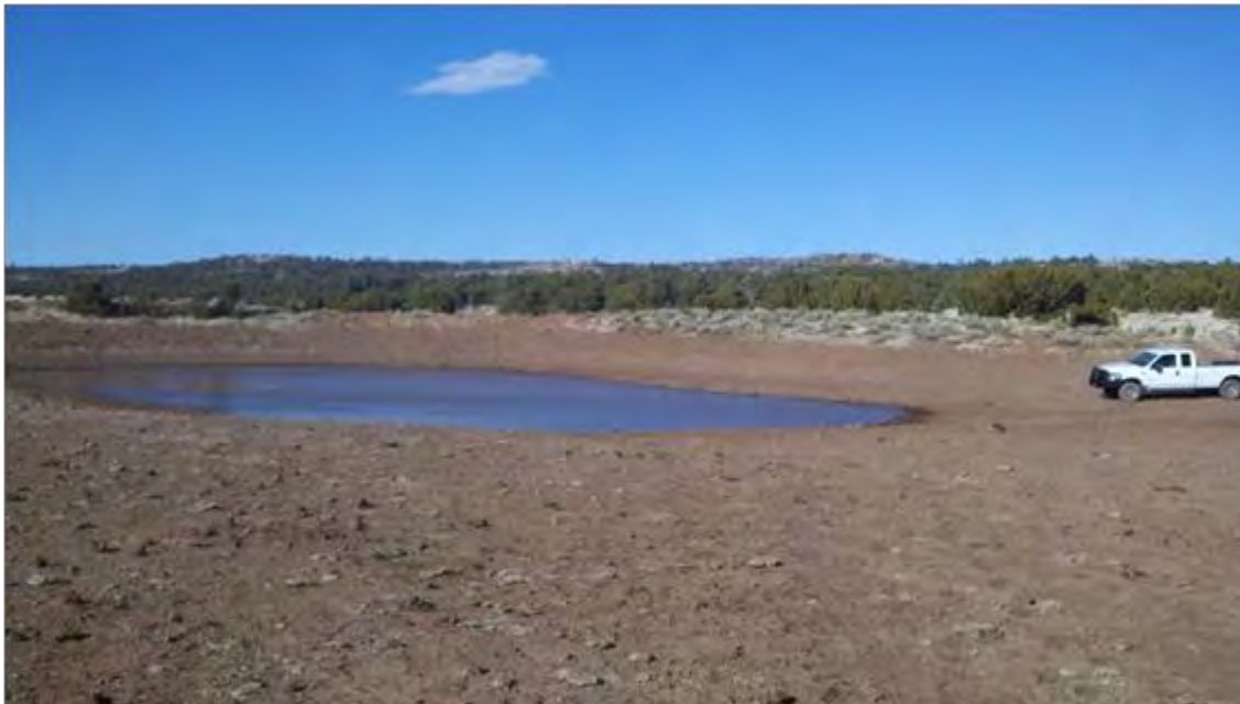
Ida Tank still holding water (Pictures taken by Copper State Earth Works, 2014).
