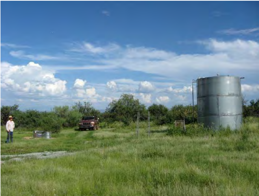
View of Storage Tank at New Well Site
