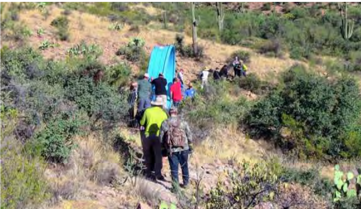
PHOTO 3; All materials and supplies are transported by hand for the Desert Bighorn Sheep Water Pipeline Project
