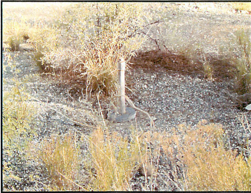
Prospect Well N350°W. Caved in well - pull or re-drill, set pump and motor.
