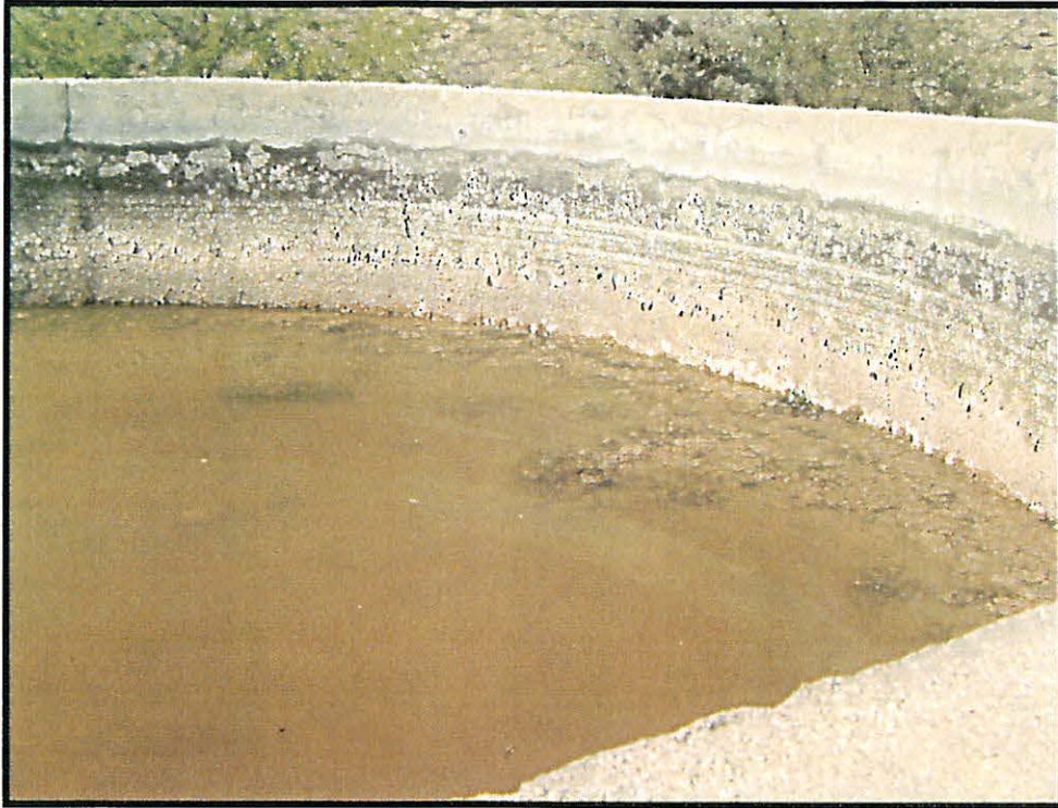
Concrete Tank #3. S200°W. Typical concrete tank for repairs, sealing, and roof installation.
