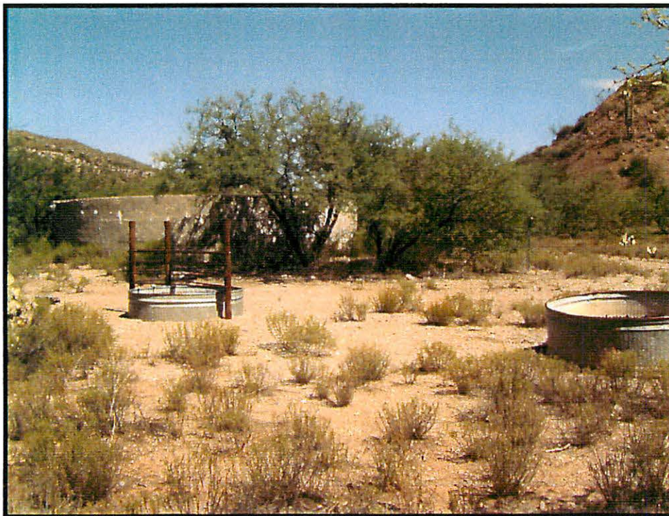
Roble West concrete storage tank. N323°W. Typical concrete tank repair, sealing and roof.
