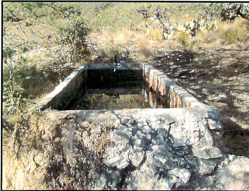
Spring Trough. S193°W. Re plumb trough and water line to new storage.
