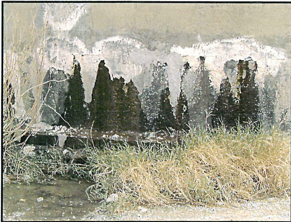
Leak in Tank #1. N32°E. Typical concrete tank repairs needed.
