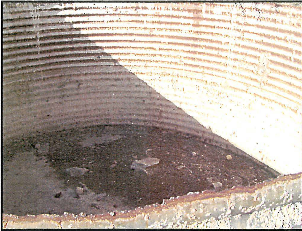
Seep Tank well S204°W. Existing tank needs repair.
