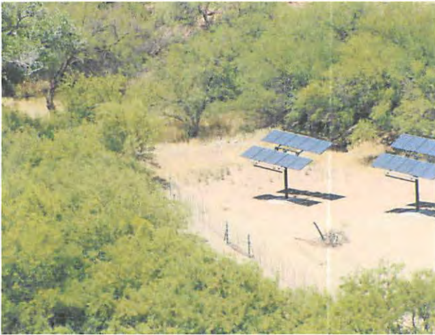
Solar installation being completed with an ADEQ and ADA grant on the Kaler Ranch
