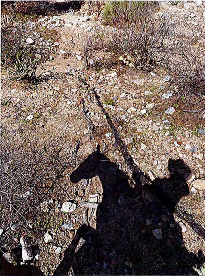
Burnt pipeline (photo above)
